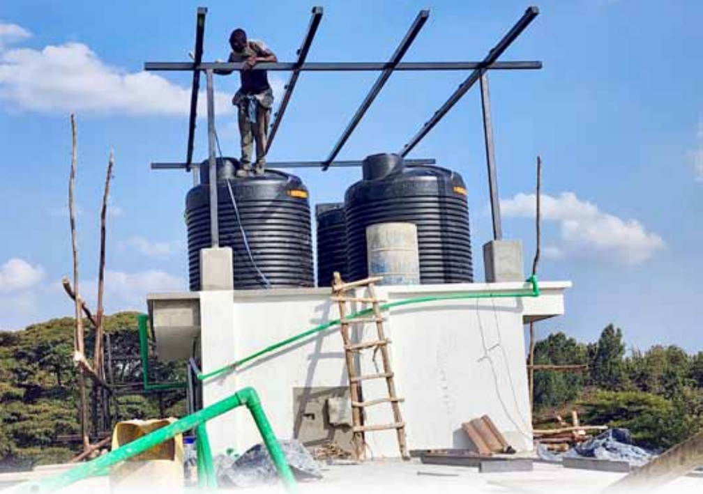
Solar structure for water tanks at Karen residence
